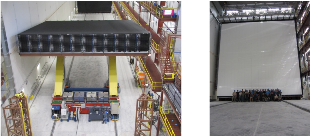
Figure 4: (a) One of 28 Far Detector Blocks is moved into position with the Block Pivoter. (b) A Block is in its final position. The installation crew of 38 people sets the scale perspective. The outside surfaces of Blocks are painted black to prevent external light from passing through the PVC material and being sensed by the APDs.
